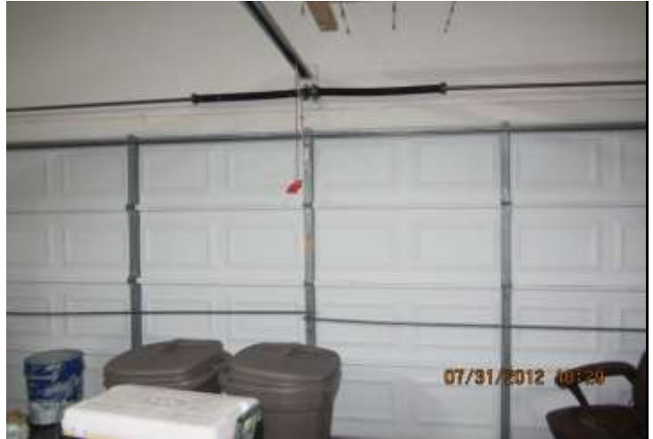
Inside of Non-Glazed Garage Door Unrated Non-Glazed Garage Door
