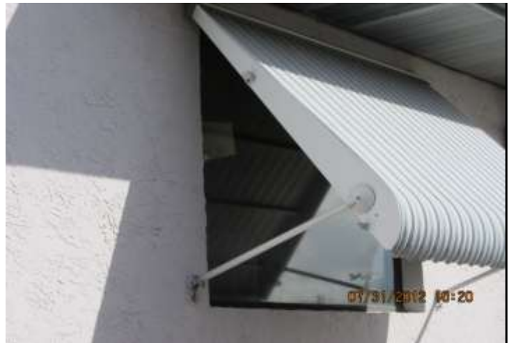
Unprotected, Unrated Glazed Openings with Non-Rated Clamshell Protection
