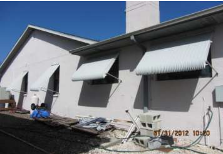
Unprotected, Unrated Glazed Openings with Non-Rated Clamshell Protection
