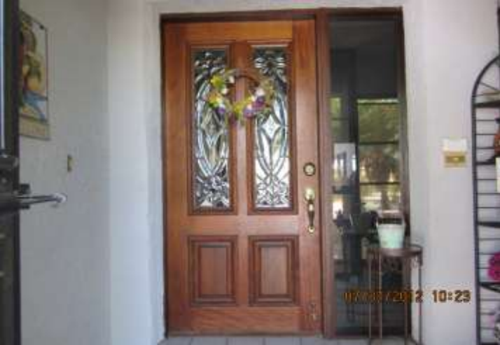
Opening Protection Unprotected, Unrated Glazed Entry
